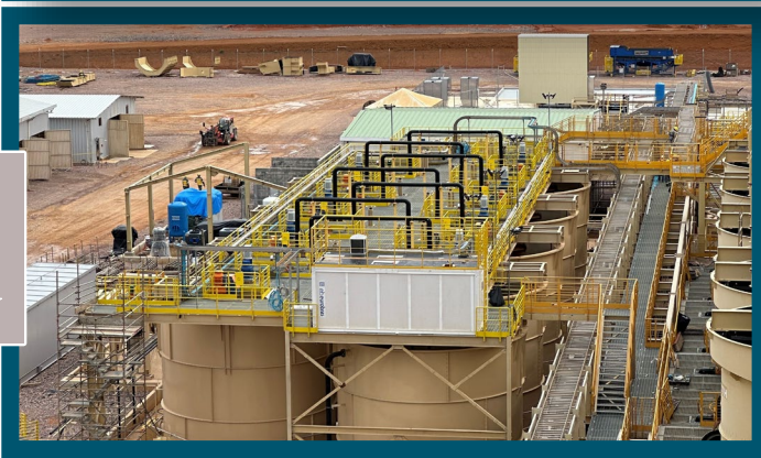
CIL Tanks 碳浸出设备
